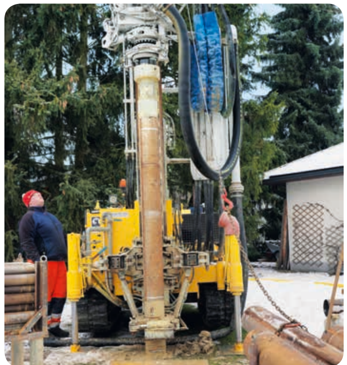
17 bar of a possible 24 bar positive pressure were enough to drill down to a depth of 60 m.
